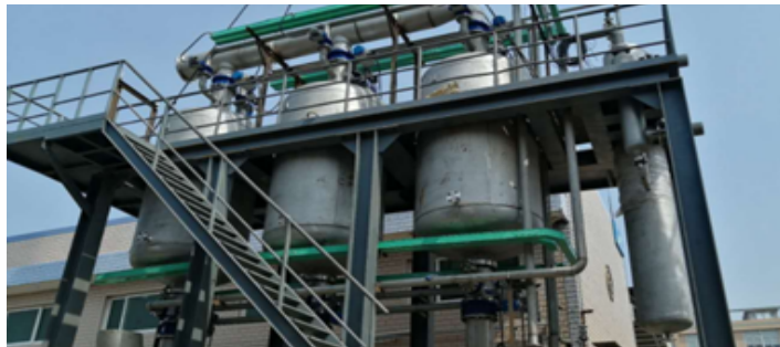
Toluene treatment project, Zhejiang (10000m 3 /h)
