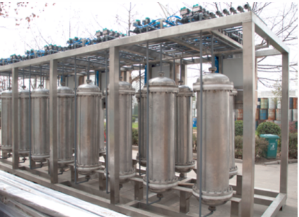
Lohexol treatment line in Zhejiang(11.25m³/h)
