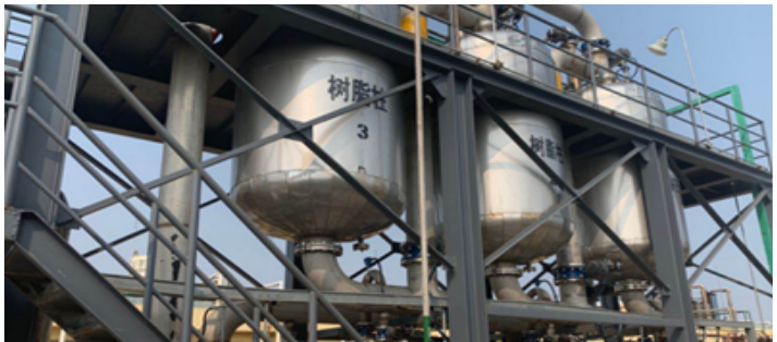
Chlorobenzene waste gas treatment project, Jiangsu
